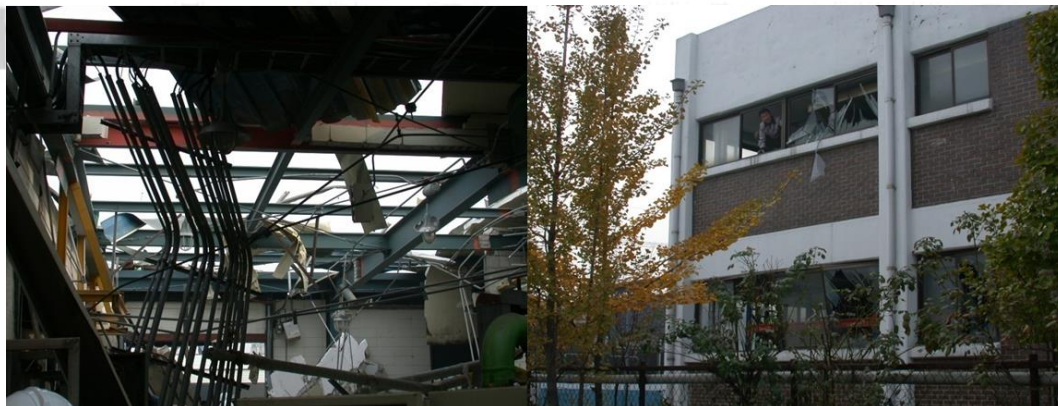
Figs. 7 & 8: Damaged Ceiling and Windows Blown Out 100 ft Away
