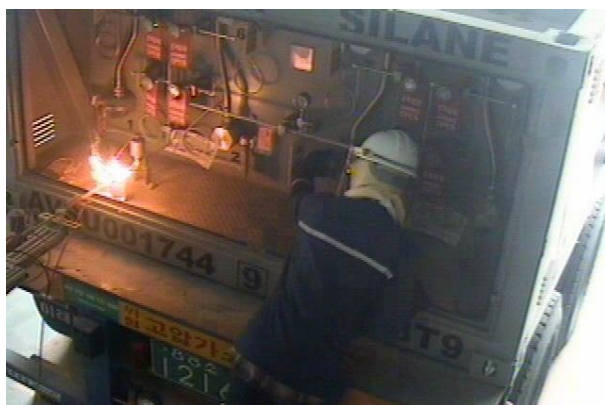
Figure 16: DISS Connection leak caused by cold liquid silane
