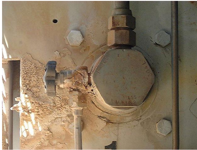
Fig. 17: Silane ISO DISS Leak
