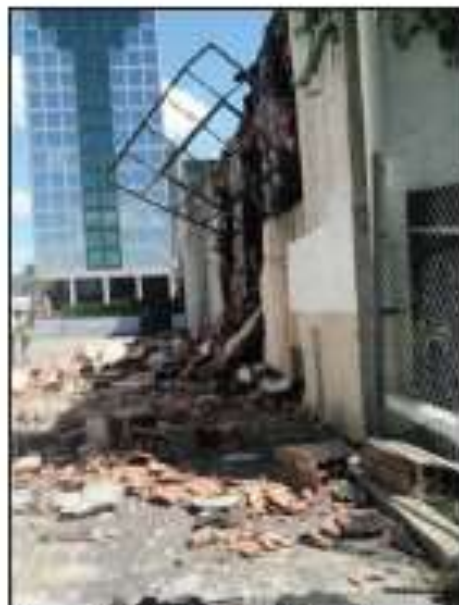
Figure 1: Exterior Wall Damage (Photo courtesy R. Sillip)
