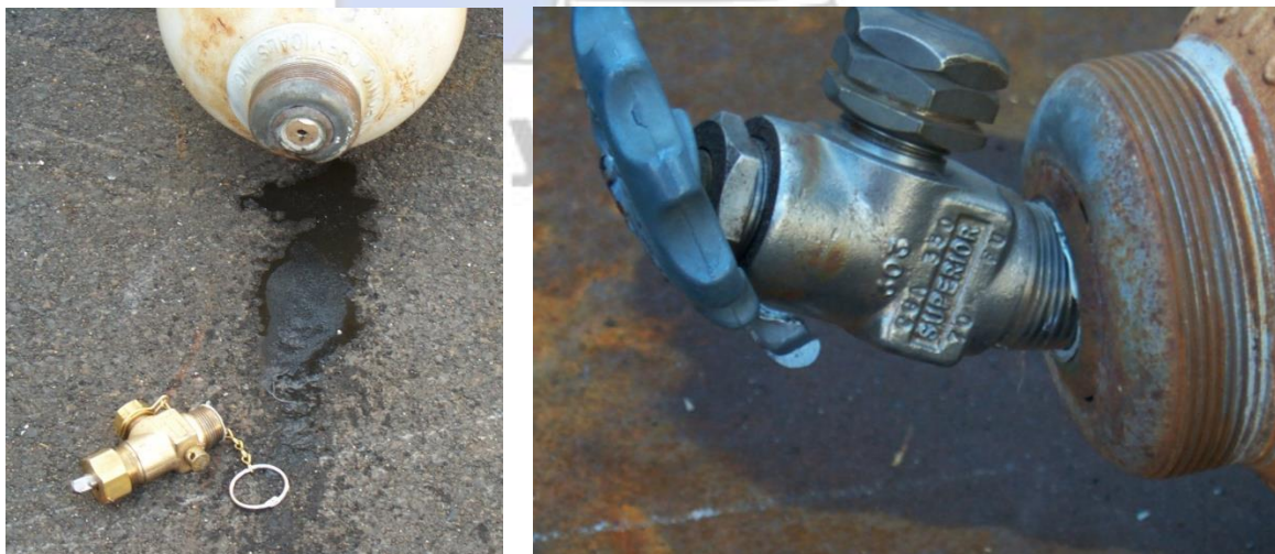
Fig 19 &20: ASB and stainless steel valves
